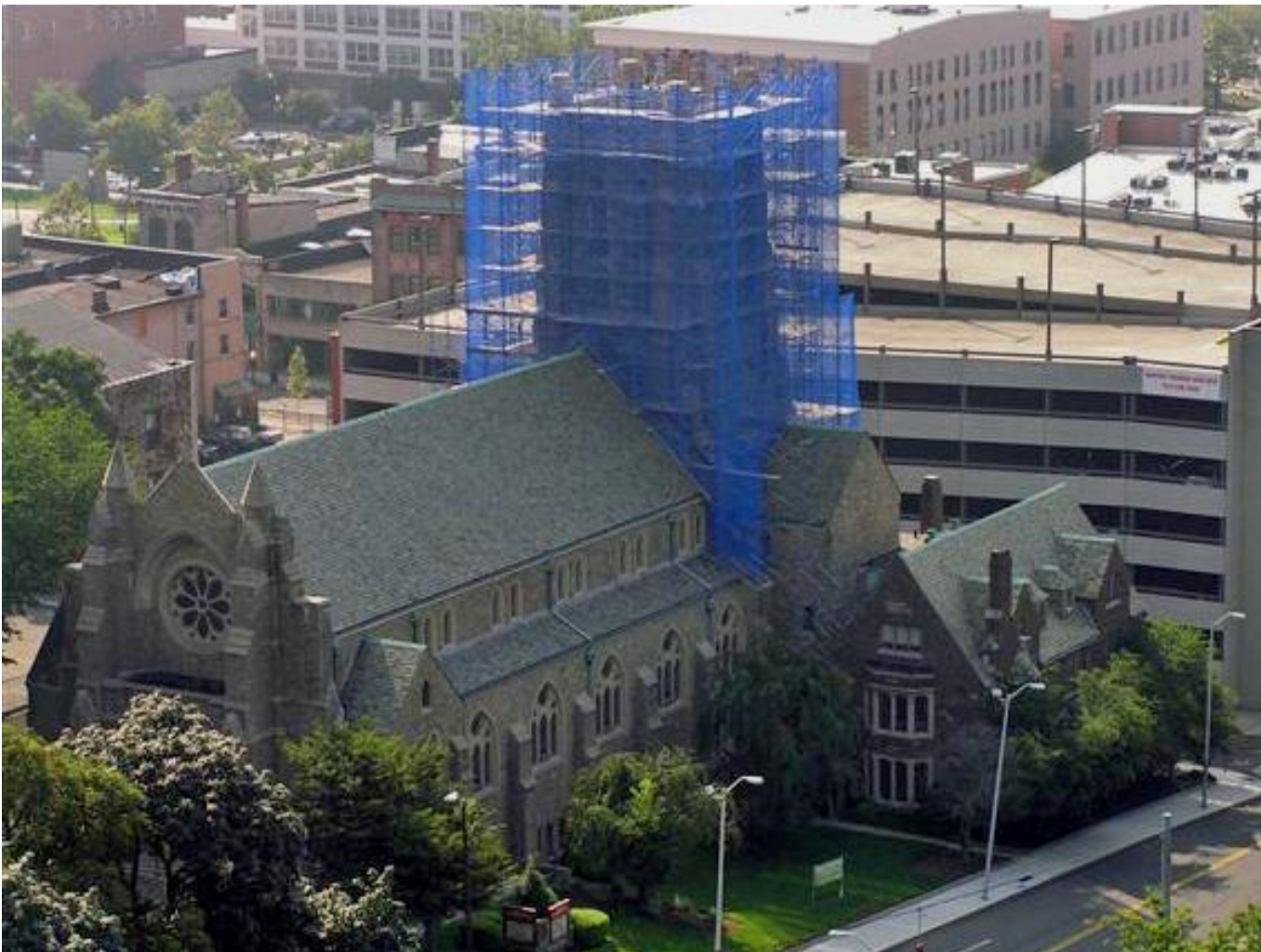
Golden Hill UMC and scaffolding around the church tower as viewed from St. Augustine Church in August.
