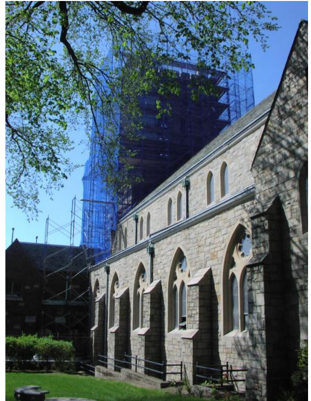
View from Golden Hill Street upper parking lot of scaffolding around the church Tower.
