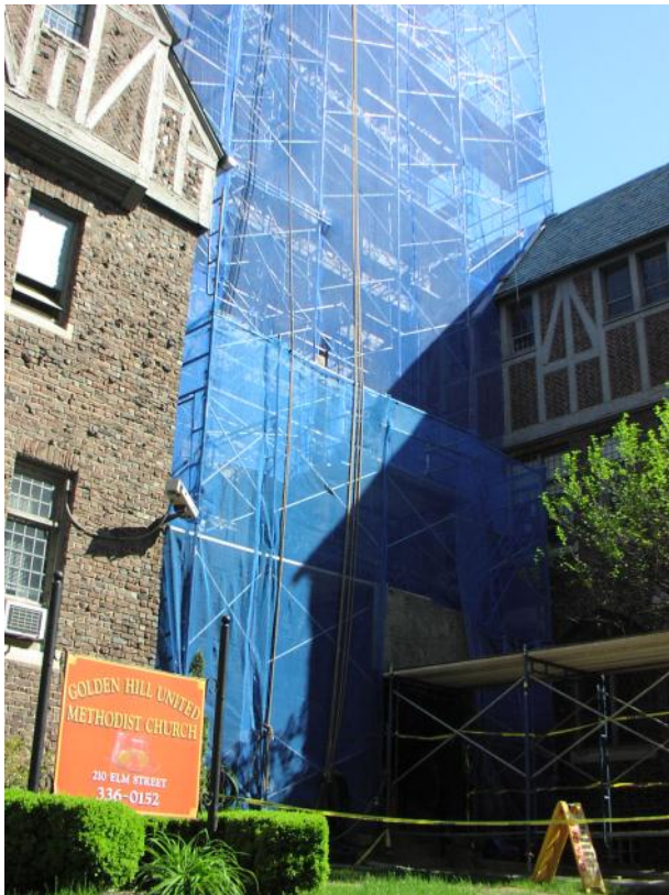
View from Elm Street of building renovation progress on the church Tower.
